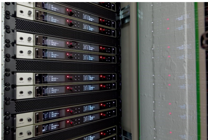
The inside of the cabinet with the EM 6000 microphone receivers. The signals are picked up by A 5000-CP passive antennas with circular polarisation
